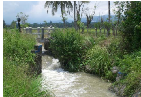
Photo 2. The condition of the structure, the primary channels of Baro Kiri (phot. A. Azmeri)
