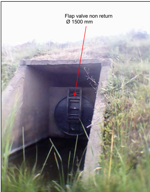
Photo 1. Downstream rejection structure of the canal towards wadi El Kebir (phot. F. Sennaoui)
