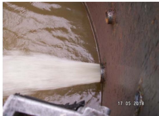
Photo 3. The mixing system in the reactor – pressing of the inert agent during the tightness test (phot. G. Walowski)
